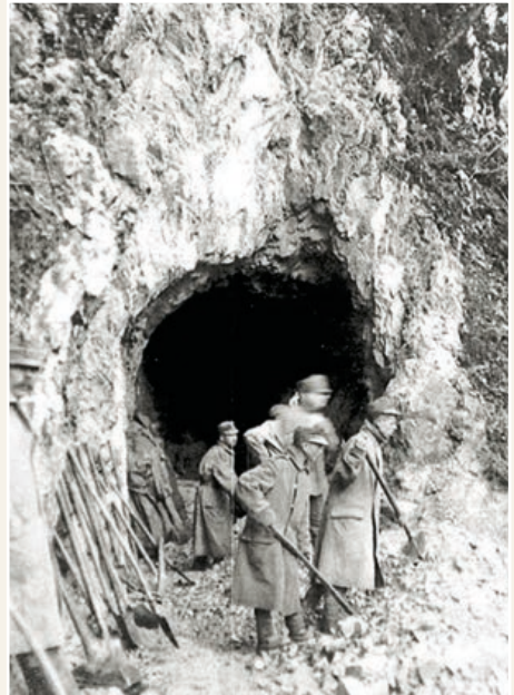
Construction of a tunnel on the route of the motorised narrow-gauge railway in Strug
